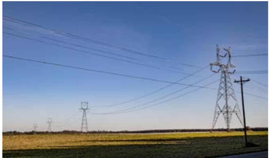
Pre-building transmission including by the local utility can send better signals to prospective resources on suitable places to connect on the system. Photo by Billy Blume, Dreamstime.
