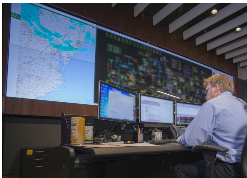
Figure 42: O&R Control Room
