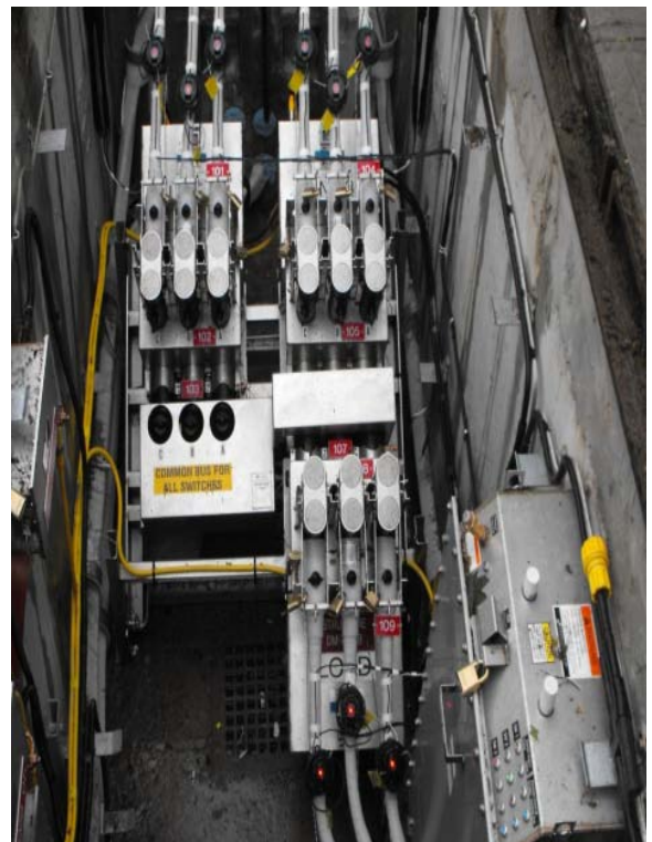
Remotely operated underground switch
