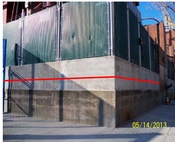
East River Substation – Red line indicates Sandy flood levels
