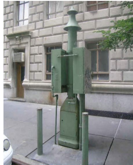
ConEdison Pressure Regulator Station
