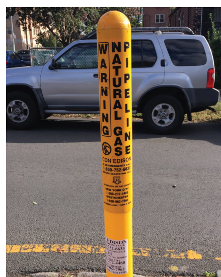
ConEdison Pipeline Marker
