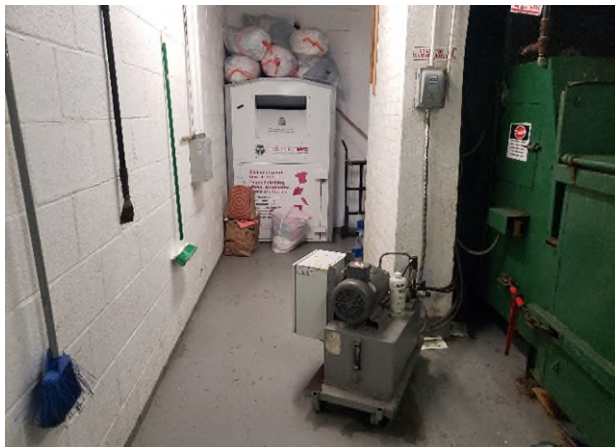
Photograph 10: Waste storage in compactor room 20 feet from HPL-Compactor Rm air sample.
