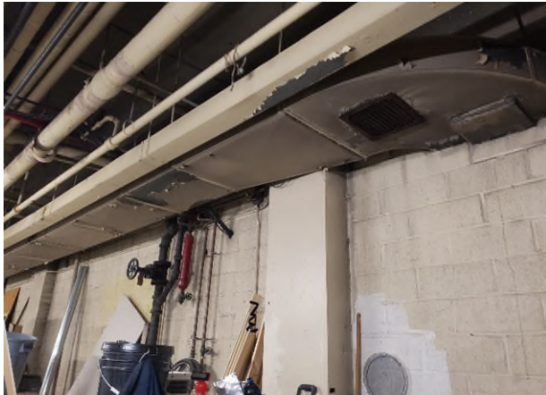
Photograph 19: Ceiling air ventilation 25 feet from HPL-Storage Rm air sample.
