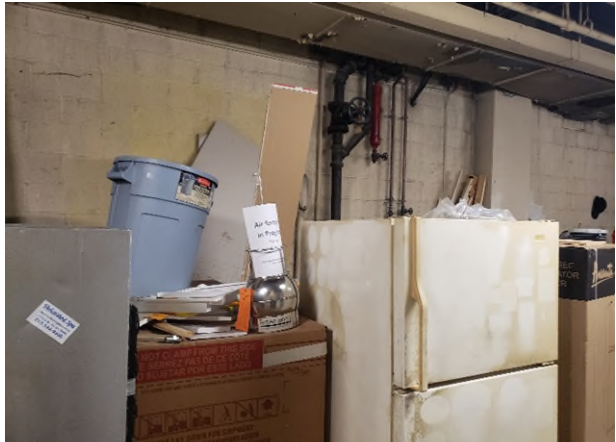
Photograph 26: HPL-Storage Rm air sample located among refrigerators 25 feet from air ventilation.
