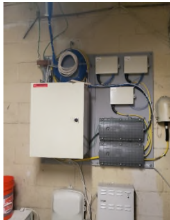
Photograph 18: Fuse box in vicinity of HPL-Storage Rm air sample.
