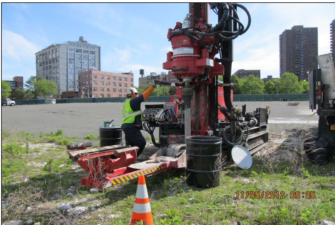
16. Start of sonic drilling activities at (new) DB-6 location in southwestern portion of Site, 5/11/12.
