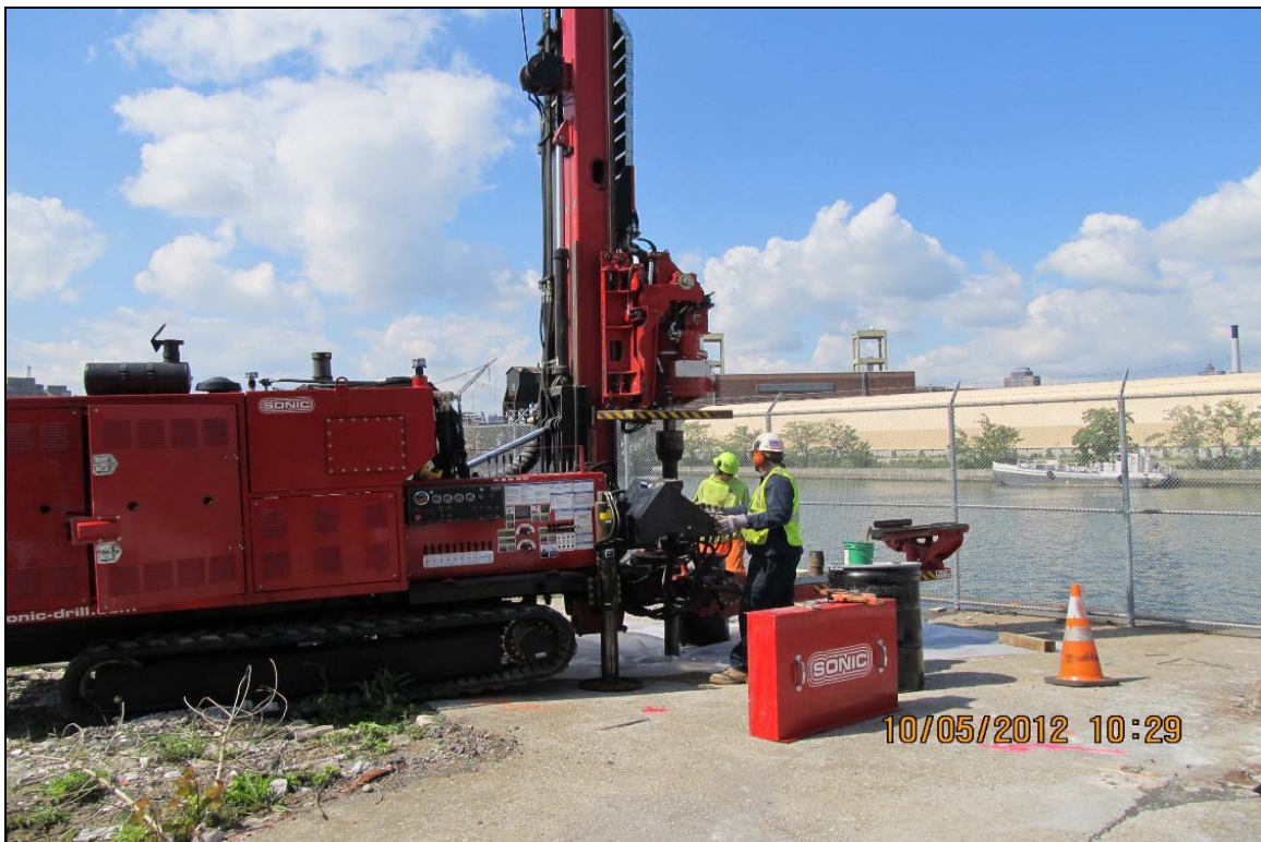
12. Start of sonic drilling activities at soil boring DB-1 location in northwestern portion of Site, 5/10/12.
