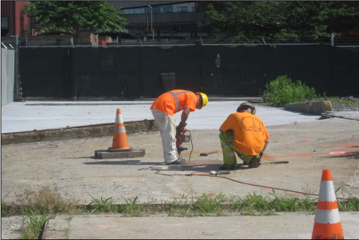
19. Installing steel plate in concrete slab over core hole and void at DB-1 location, 6/1/12.
