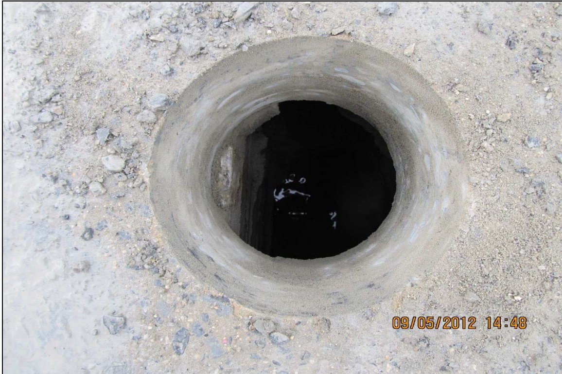
11. View of void, sub-grade structures, and water of Wallabout Channel below DB-2 location, 5/9/12.
