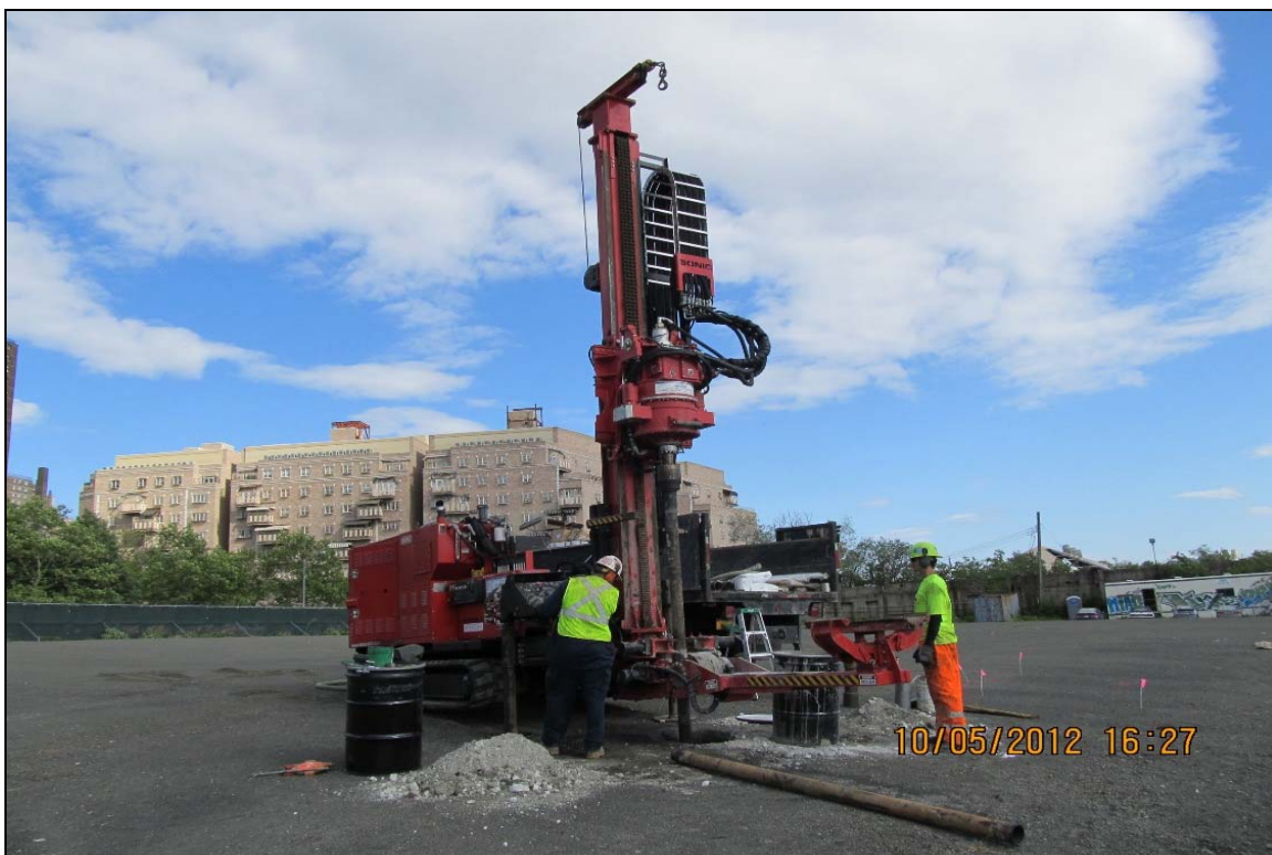
14. Sonic drilling activities at soil boring DB-3 location in west-central portion of Site, 5/10/12.
