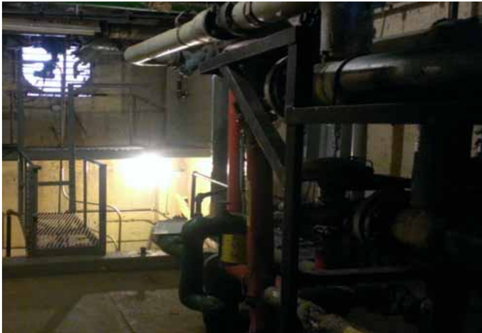
Piping units within tank room (facing east) located within 170 Avenue D.
