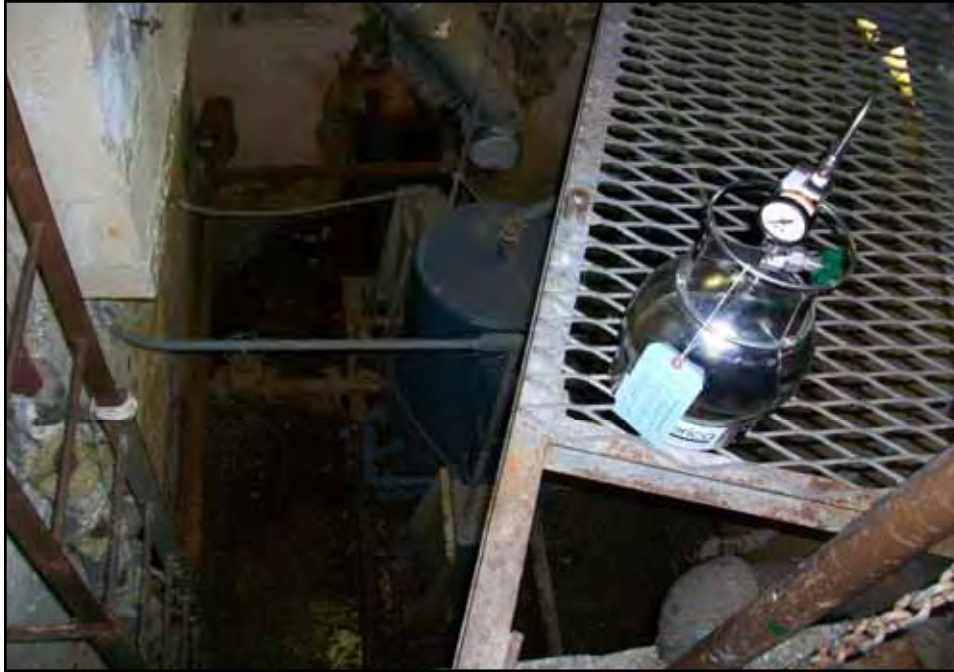
Pit and sump (with JR-1141-IA-2) within Tank Room located at 1141 FDR Drive.
