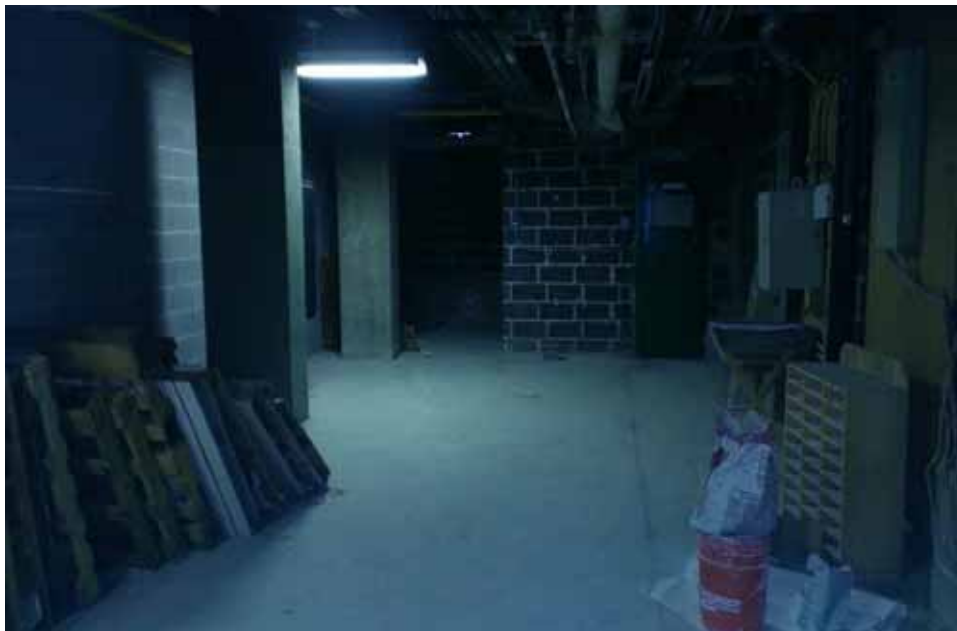
Outside of plaster room area facing meter room (south) located within 1115 FDR Drive.
