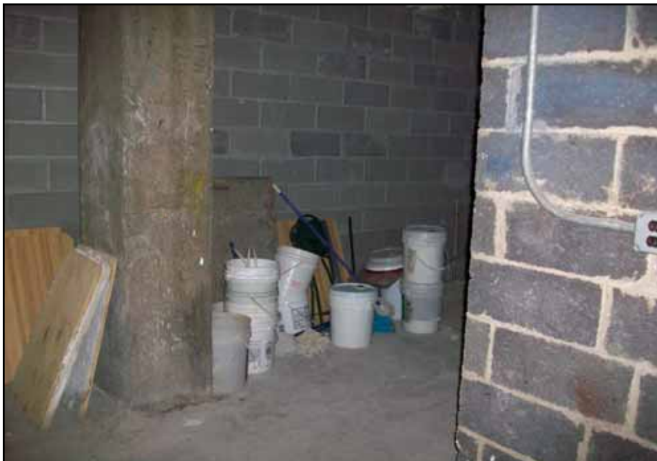
Various empty (used) cleaning buckets and cleaning solution located in plaster room within 1115 FDR Drive.
