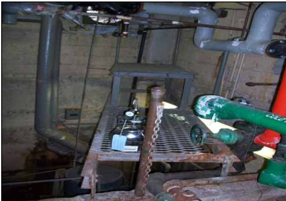
Tank room (facing northeast) containing JR-1141-IA-2 within 1141 FDR Drive. Tank room contains various piping and a pit with a sump.
