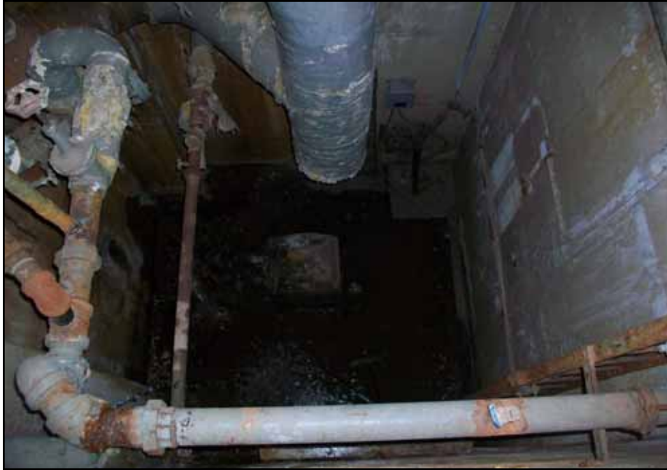
Pit and sump containing water located within tank room at 1115 FDR Drive.
