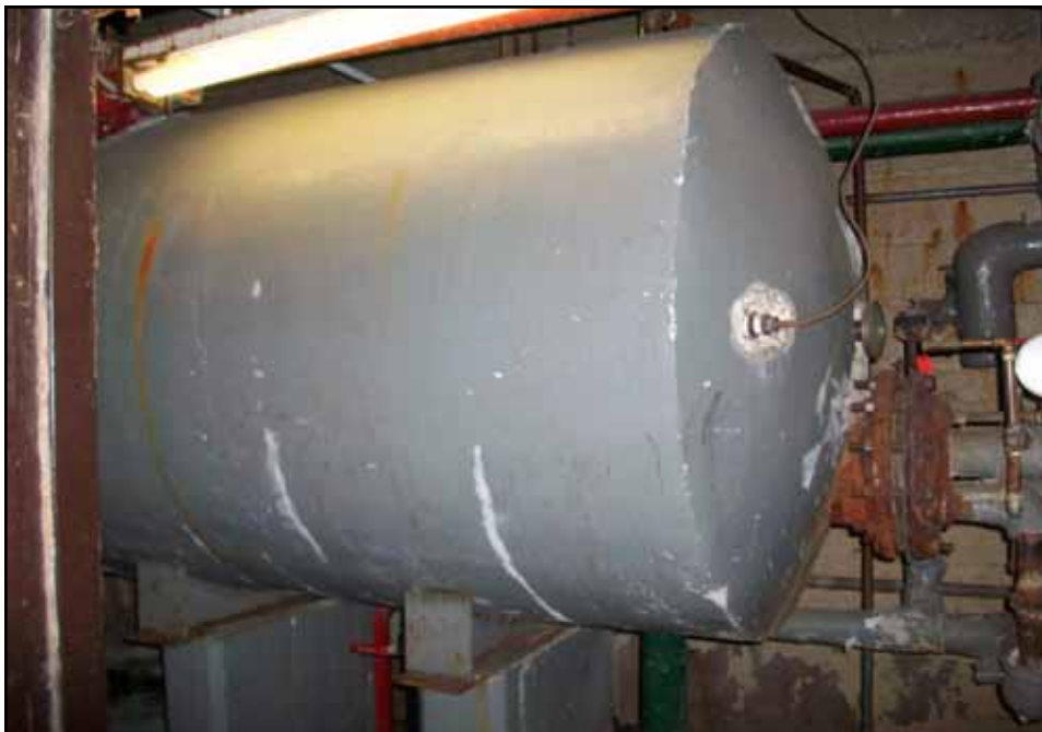
Tank room (containing 2 drains and fans) located within 1223 FDR Drive.
