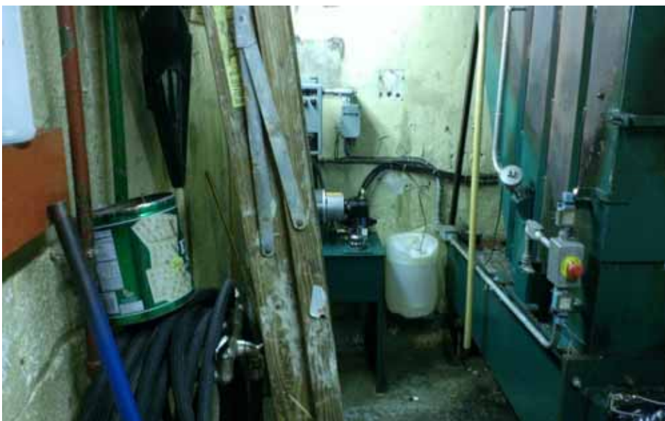
Compactor room located in 170 Avenue D containing Bio-Wash for trash compactor unit and oil-containing unit for compactor operation.
