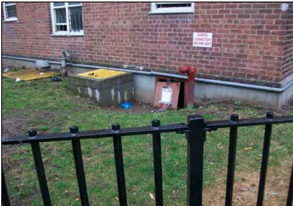
Vault with crawl space (facing east) where JR-178-IA-1 was located at 178 Avenue D.
