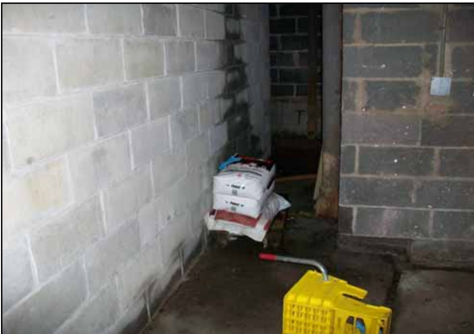
Outside of storage room (facing south) containing bags of rock salt and a mop bucket within 1223 FDR Drive.
