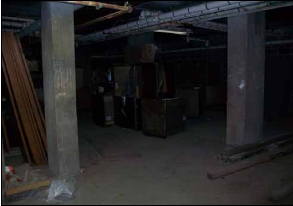
Storage room area (facing east) where JR-1115-IA-1 was obtained within 1115 FDR Drive.
