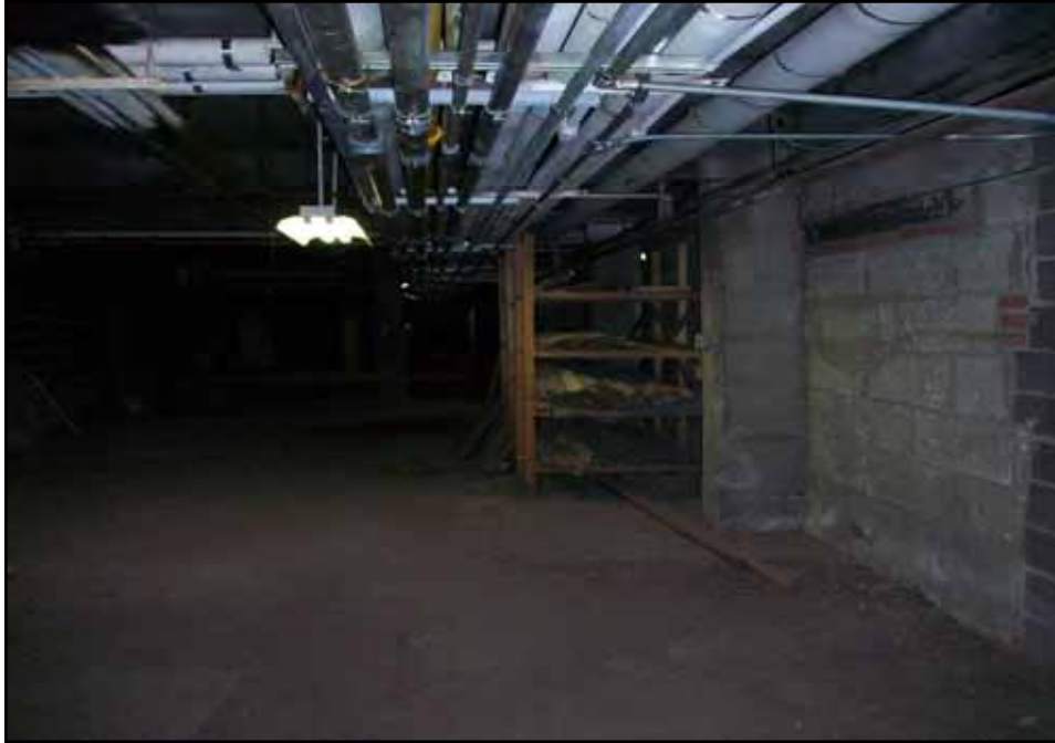
Main walkway (facing east) containing various building-related materials located within 1223 FDR Drive.
