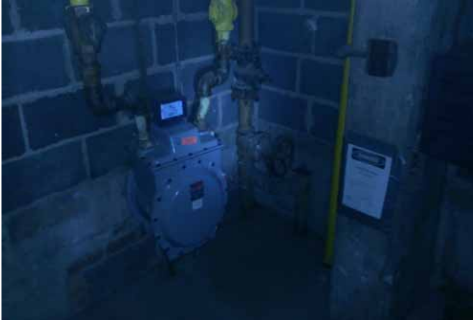
Meter room (facing west) located within 178 Avenue D.
