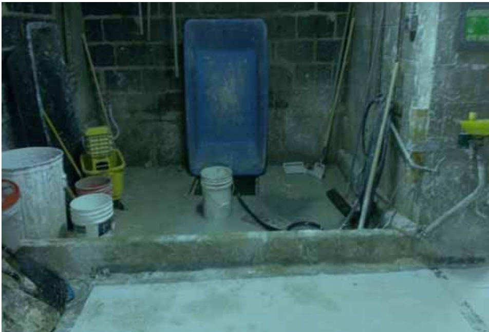
Grout mixing area plaster and adhesives located in plaster room (facing south) within 1115 FDR Drive.
