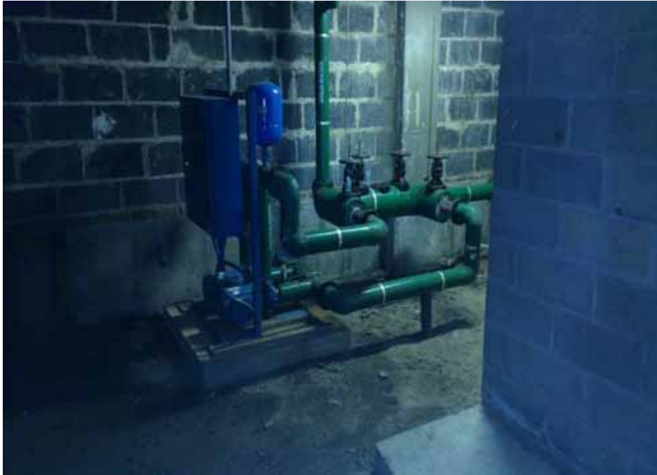
Assorted piping (facing east) contained outside of telecommunications room (on right) within 1223 FDR Drive.
