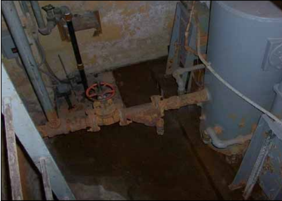
Pit with sump located in tank room (facing east) within 170 Avenue D.
