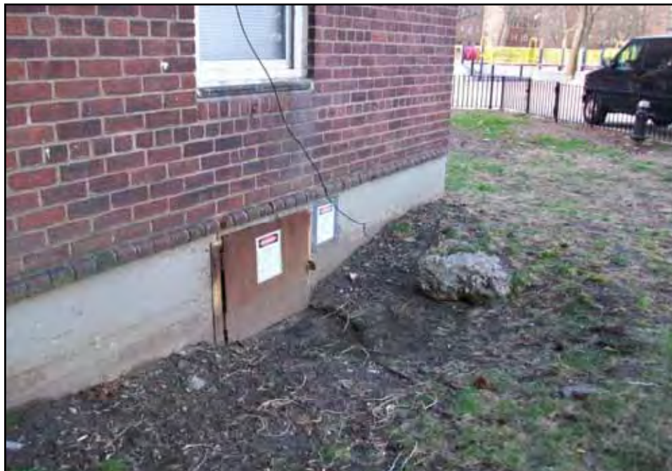
Vault containing crawl space (facing south) where JR-1141-IA-1 was located at 1141 FDR Drive.
