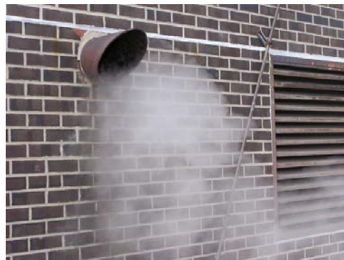
Figure 5: Relief valve leaks are usually overlooked, but can result in significant increases in steam consumption.
