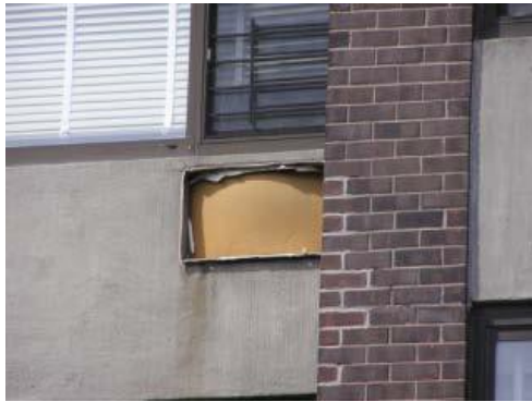
Figure 12: Poor building envelope maintenance, as exemplified by this missing AC sleeve cover, contribute to increased energy consumption.
