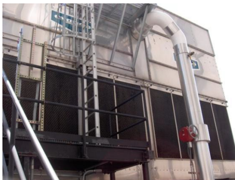
Figure 11: To maximize resource recovery, condensate can be used for cooling tower make-up after its heat has been recovered.
