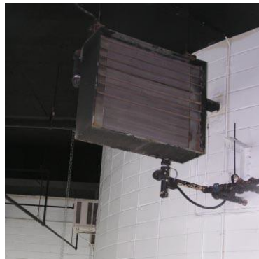
Figure 17: Minimizing the use of non-essential heating, such as this garage heater, during the on-peak period will help reduce demand.
