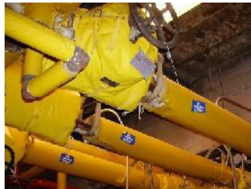
Figure 3: Insulated valves with removable jackets.
