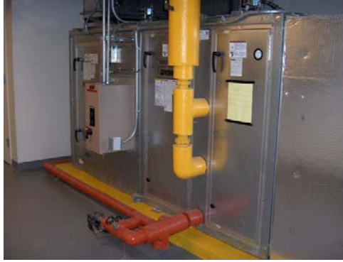
Figure 18: Starting up air handling units before 6:00 a.m. or staggering their start-up will reduce the on-peak demand.
