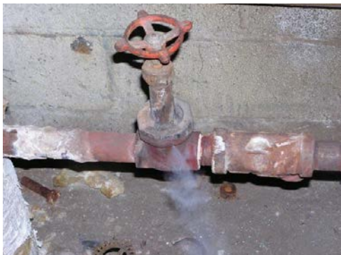
Figure 4: Investing the capital to fix visible steam leaks typically results in a high ROI.
