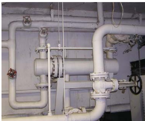
Figure 9: A condensate heat recovery system with a shell and tube heat exchanger.
