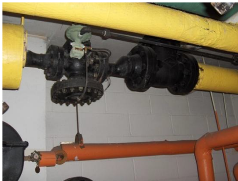
Figure 2: Un-insulated PRV and shut-off valve.
