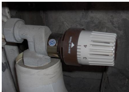
Figure 7: Thermostatic radiator valve.
