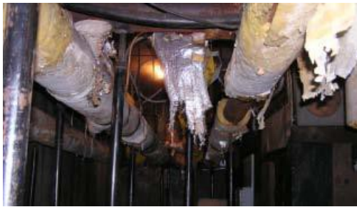
Figure 1: Missing piping insulation.
