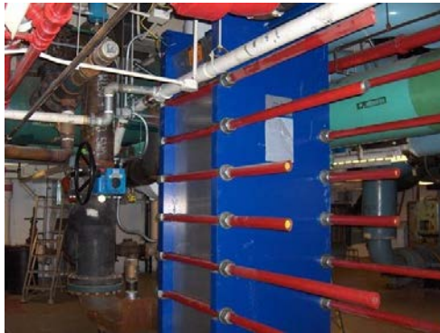
Figure 8: Plate and Frame Heat Exchanger.
