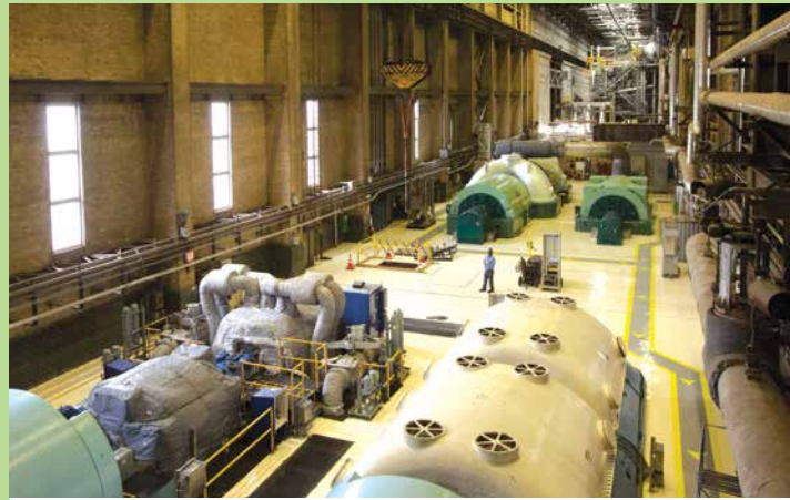
Con Edison Congeneration Plant
